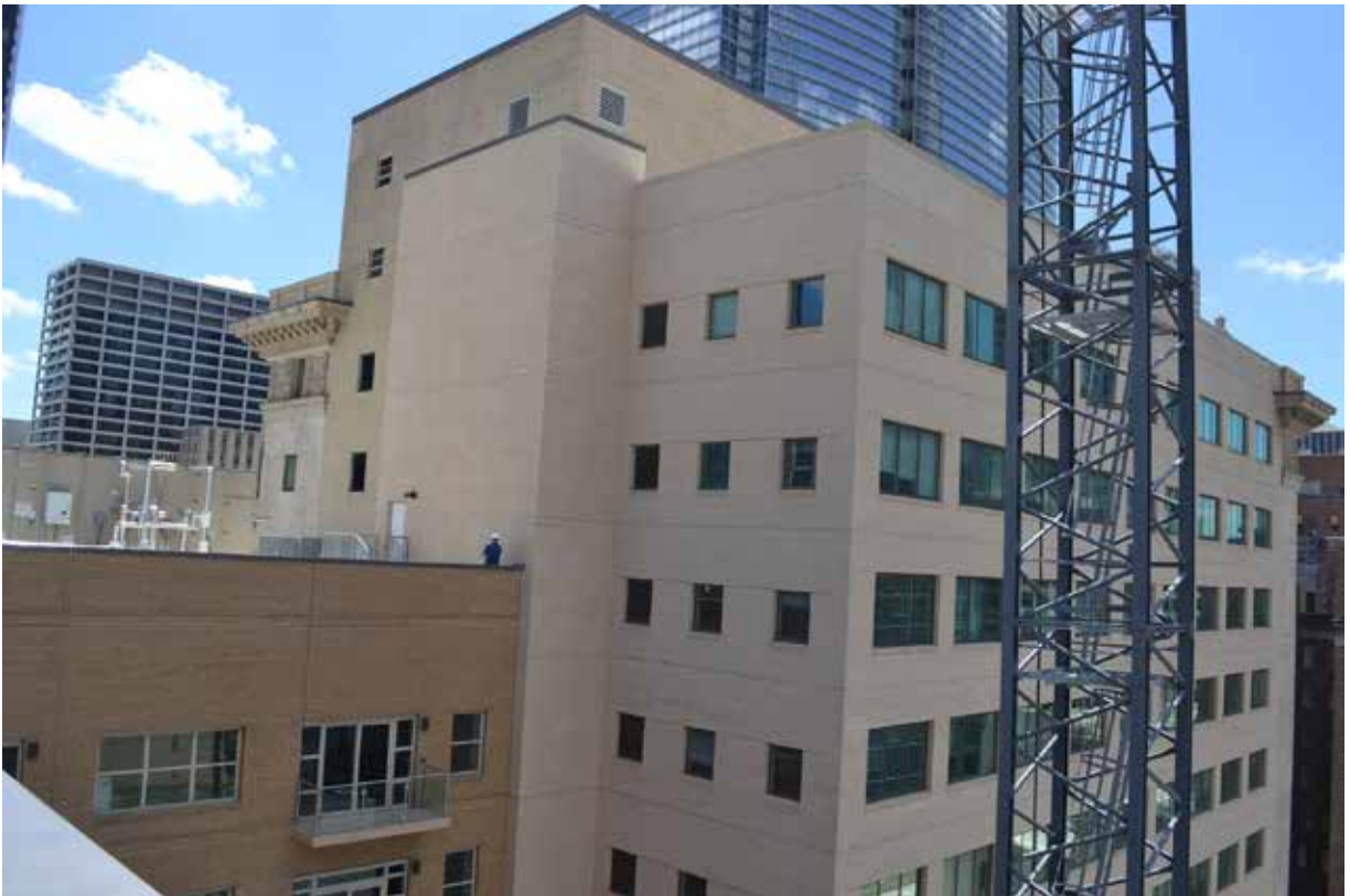
B: Roof, view SW from 1936 roof of new fire stair and rebuilt 1959 N wall June, 2017
