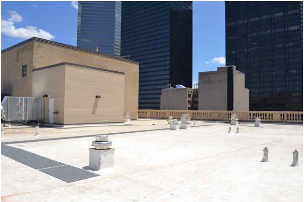
B: Roof, partial N and W elevations of 1959 penthouse, view SE June, 2017
