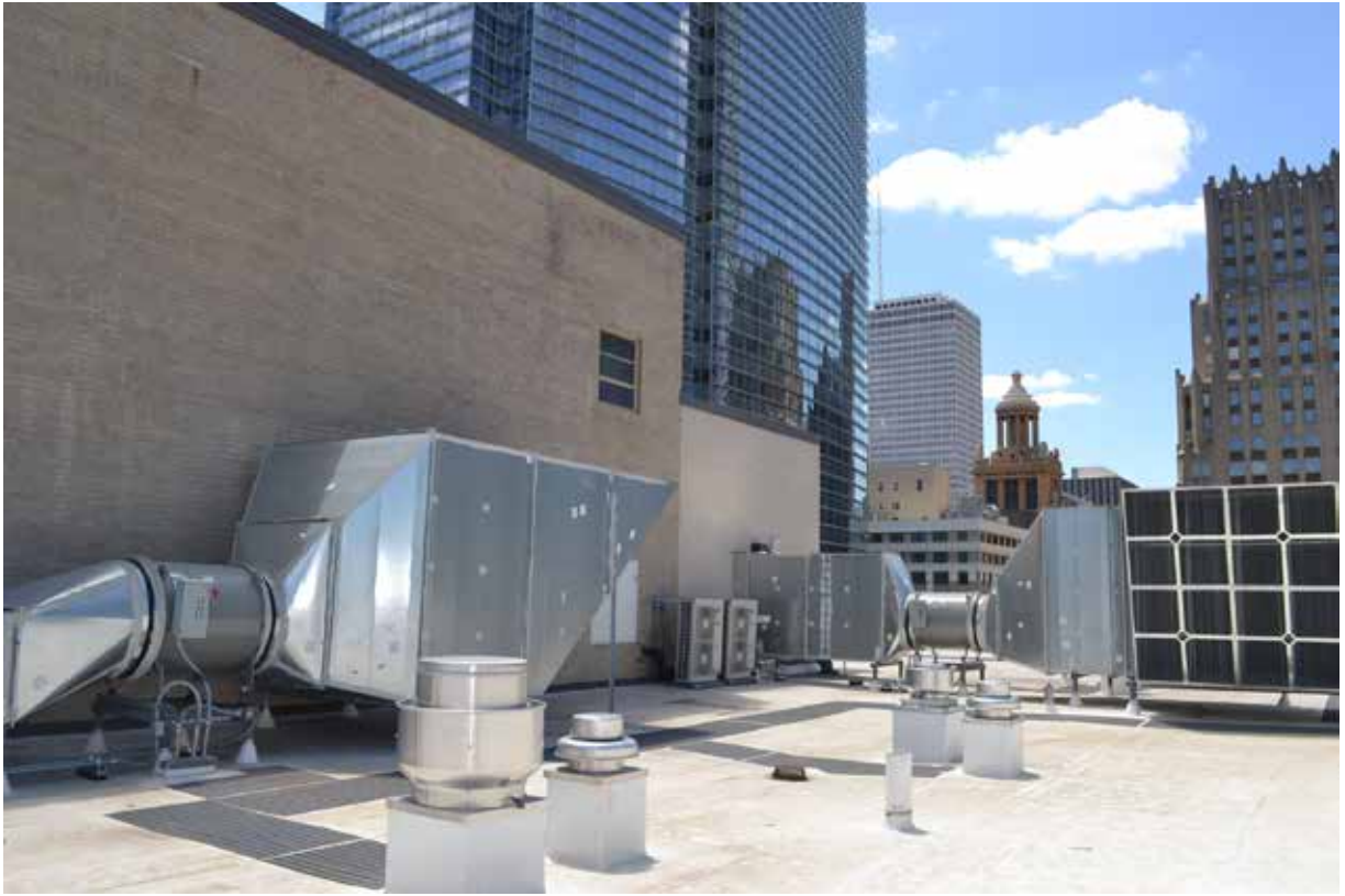
A: Roof, N elevation of 1959 penthouse and new stair pressurization equipment, view SW June, 2017
