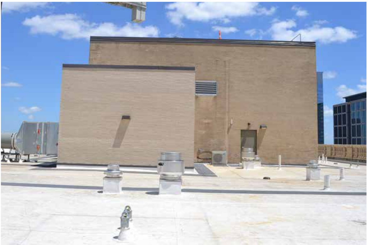
B: Roof, W elevation of 1959 roof penthouse (in rear) & new mechanical addition, view E June, 2017
