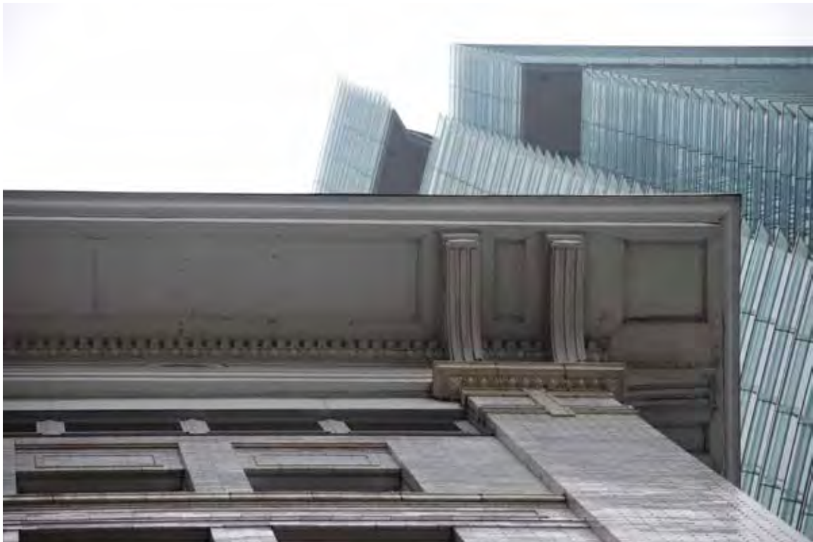
B: Detail of glazed brick, pilaster capital, and cornice. SWCA photo, 2014. File: 00_DSC_0162
