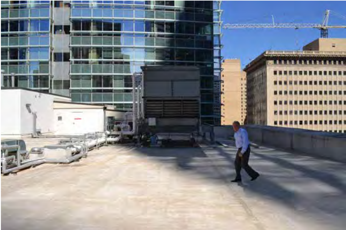
A: Roof, view N from SE corner. Mechanical penthouse and electrical closet on L. SWCA photo, 2014. File: 0667
