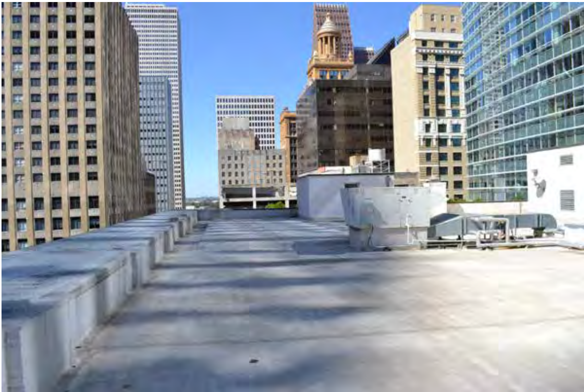
B: Roof, view W from SE corner. Old elevator penthouse behind HVAC unit. SWCA photo, 2014. File: 0669
