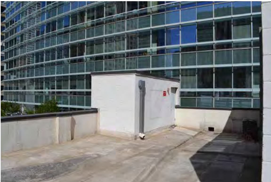
B: Roof, view NW of south (L) and east (R) elevations of stair penthouse. SWCA photo, 2014. File: 0676
