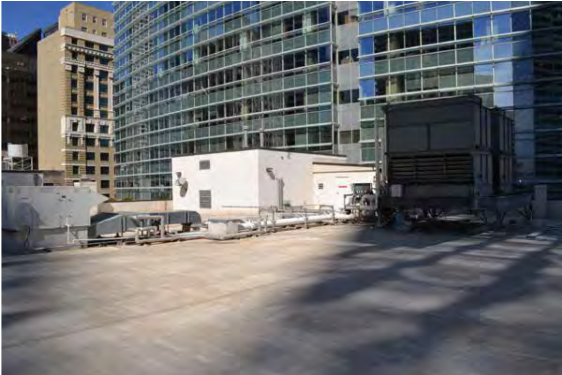
A: Roof, view NW from SE corner. Mechanical penthouse (L), electric closet (R). SWCA photo, 2014. File: 0668
