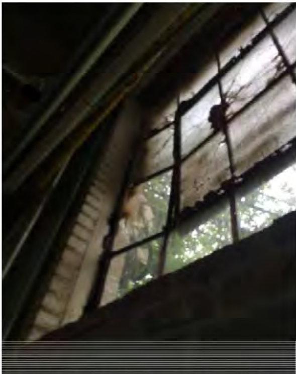
EXAMPLES OF SEVERE DAMAGE TO EXISTING HISTORIC STEEL WINDOWS
