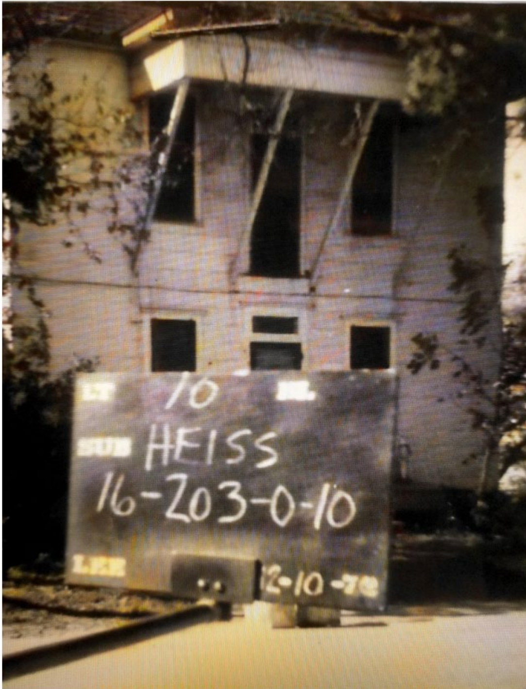
Subject property in 1972. Porches had rotted/been removed.
