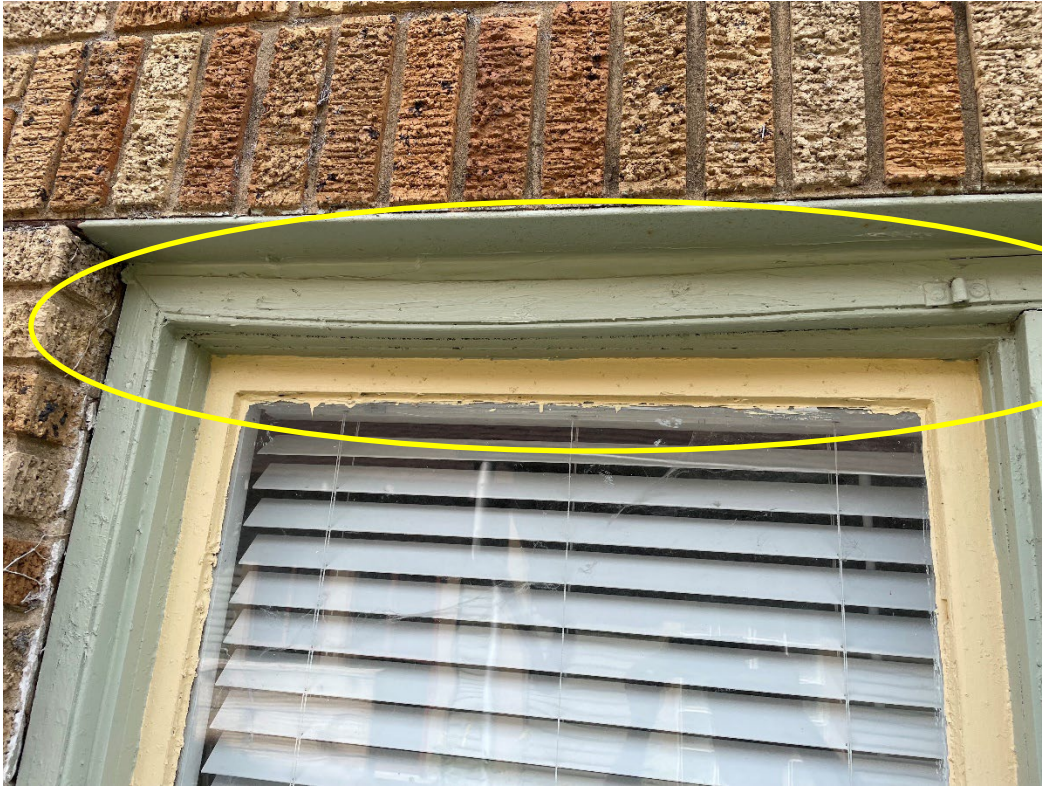
Figure 1 - Original - warped brick molding
