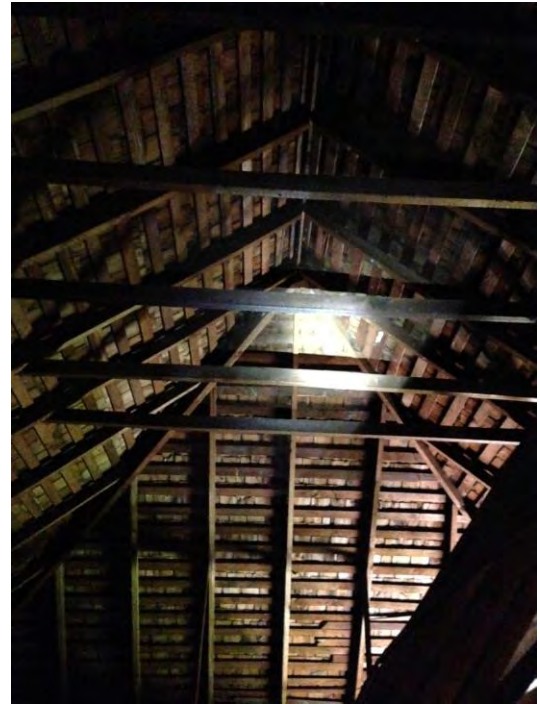
Figure 1: Unsupported Roof Hips
