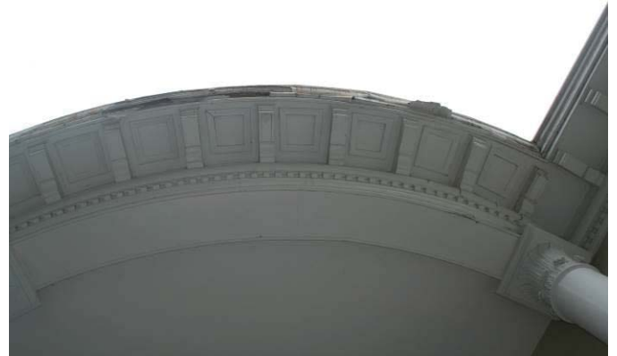
Repairs needed at Front Canopy Cornice
