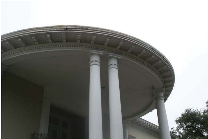
Repairs needed at Front Canopy Cornice
