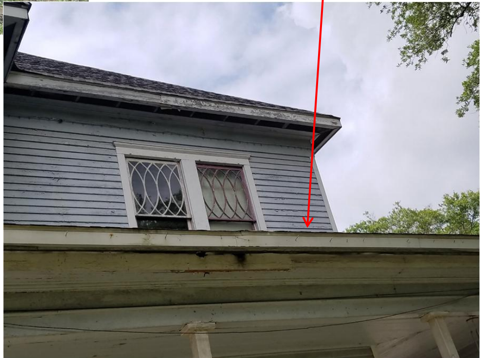
2 nd Floor Porch Previous owner replaced 2 nd floor porch with plywood and shingles
