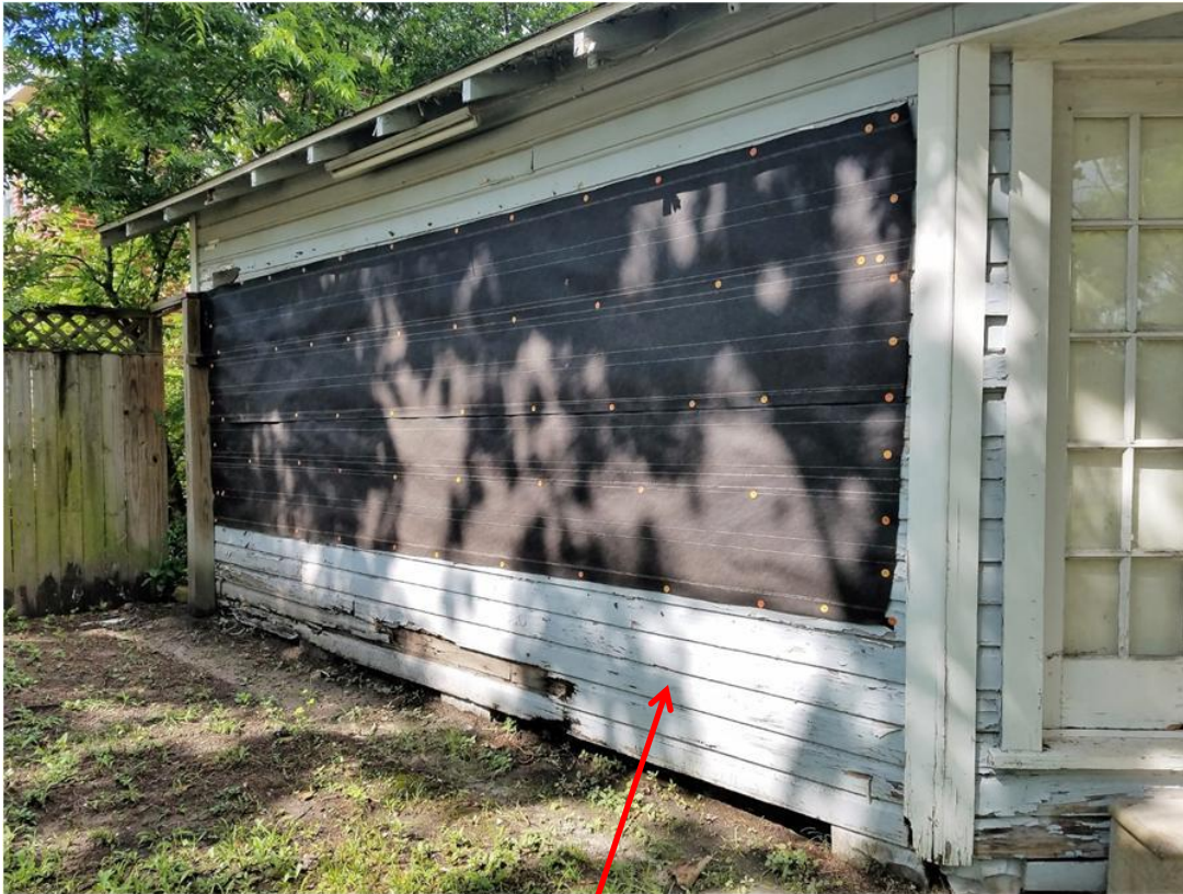
Flower Shop (facing Beauchamp St.) Existing site of 1-story addition (former flower shop); renovation plans propose this location to be converted into a garage (Due to water leakage and ingress / egress from various vermin, we have tarped the outside of the structure as a temporary fix)
